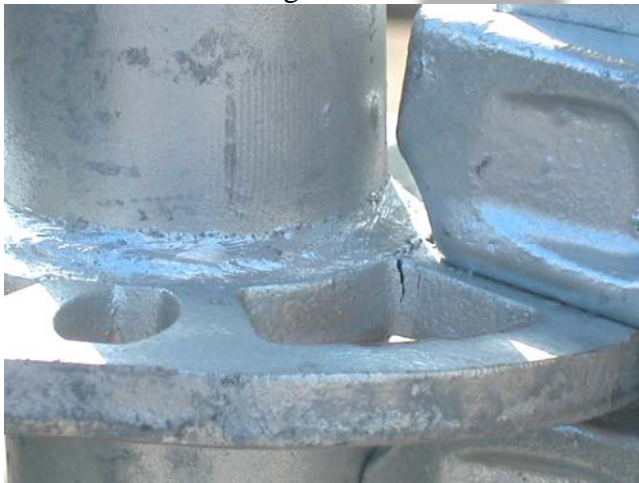
Crack in rosette, test #1 at 11,000 lbs.
